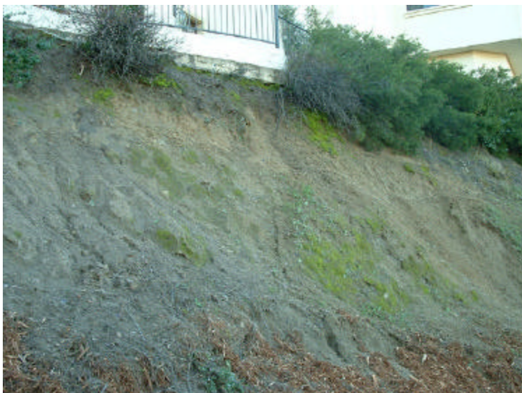
Figure 11. No erosion preventing vegetation roots have allowed ongoing damage to slope and starting to threaten foundation of structure above.
