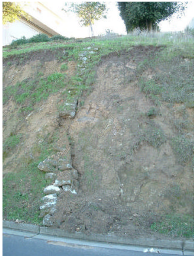
Figure 13. Nearby slide destroying pipe-covering cement filled bags.
