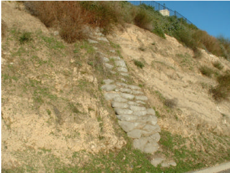
Figure 9. Unattractive cement filled bags covering drainage pipe.
