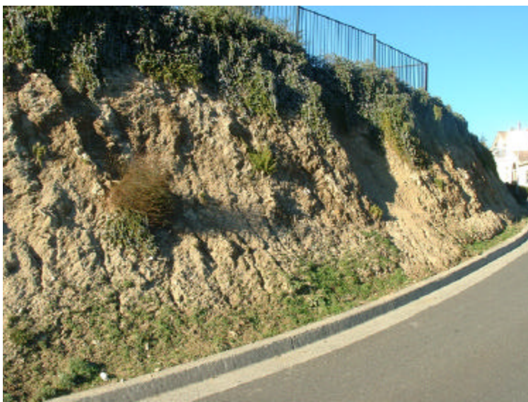
Figure 10. Exposed bedrock has been eroded and channeling is appearing due to runoff from above.
