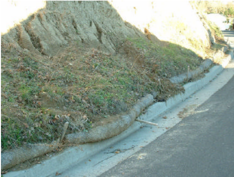
Figure 6. Slide overwhelming temporary straw pipe retaining structure. Erosion has left exposed rock with no soil remaining allowing erosion to start working on these materials.
