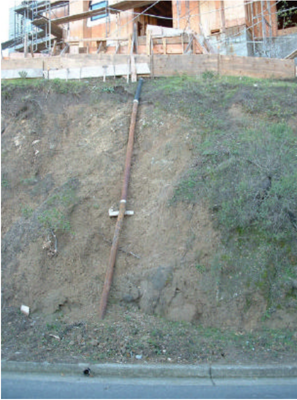
Figure 13. One of the more attractive drainage pipes the residents must view on a daily basis.
